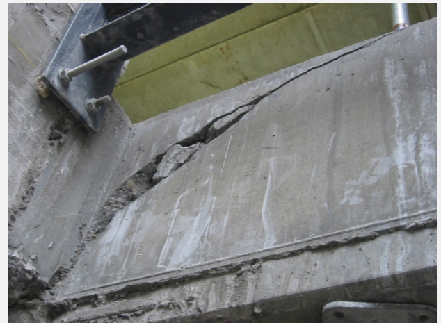
Premature shear failure in concrete slab optimized by yield line method
